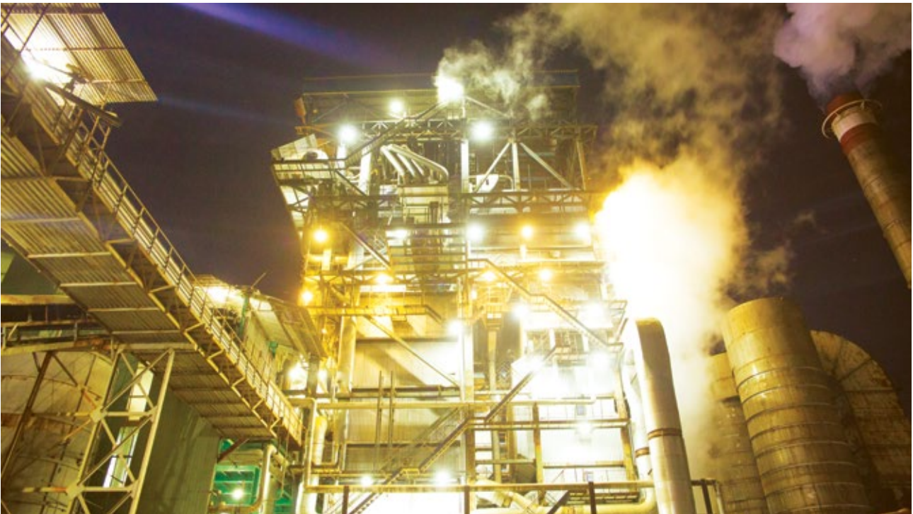
Sugar refining system using biomass fuel at Bien Hoa factory - Ninh Hoa
