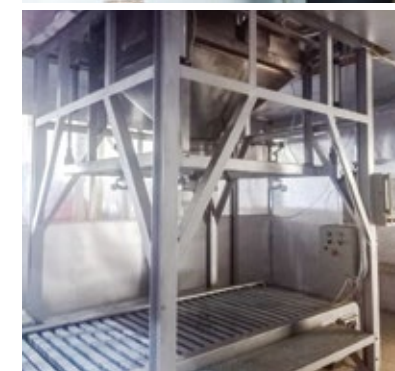
Bigbag packaging system at TTC Attapeu factory
