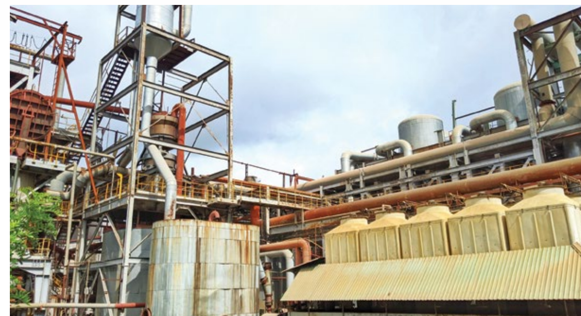
Steam saving system at Bien Hoa - Ninh Hoa factory
