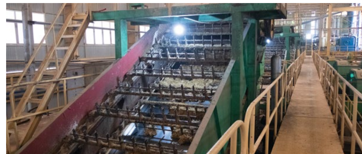
Dry sand separation system at TTC Attapeu factory
