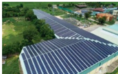
SBT's rooftop solar power system at TTC Gia Lai
